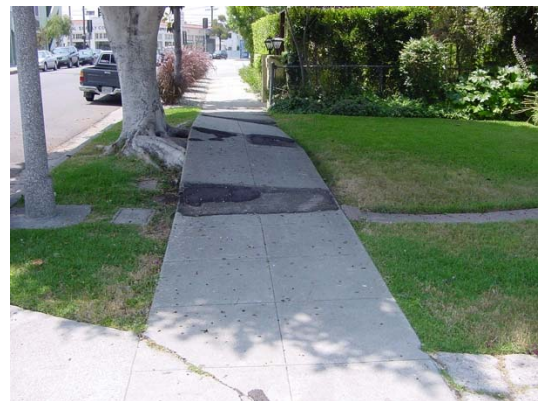
Uplifted sidewalk (Credit: Ryan Snyder)
