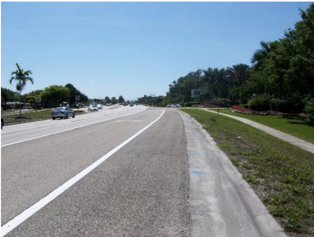
Photo 3: Full depth pavement structure needed to replace shoulder pavement structure at keyhole locations (typical).
