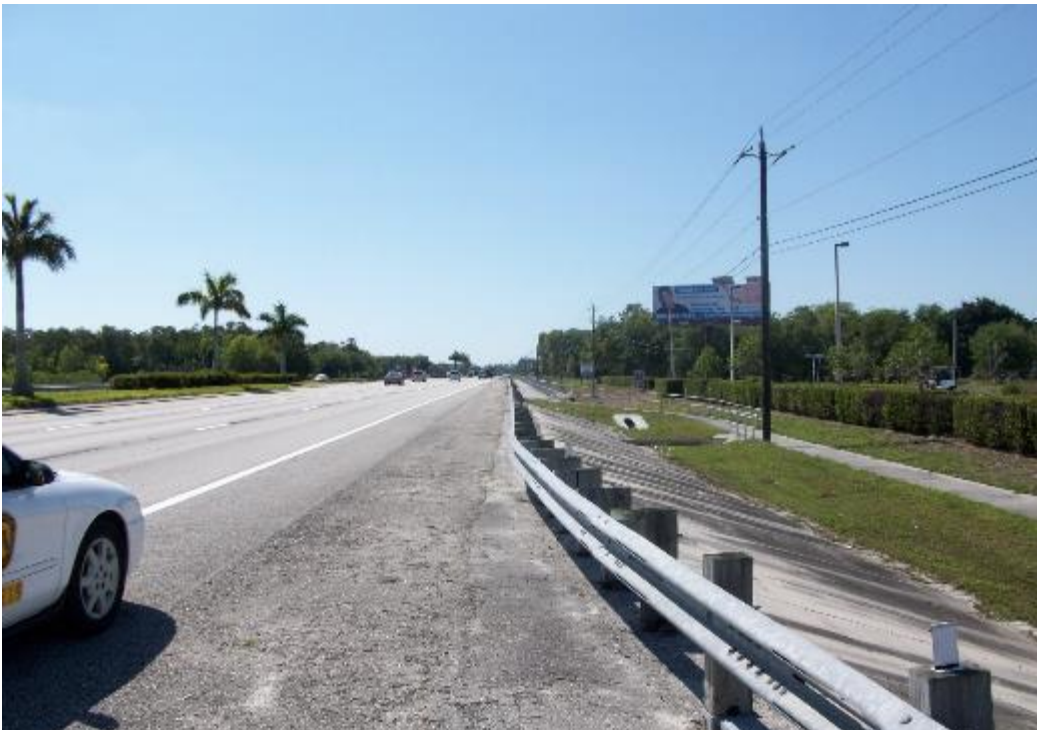
Photo 1: Mill and resurfacing required at shoulder in front of guardrail
