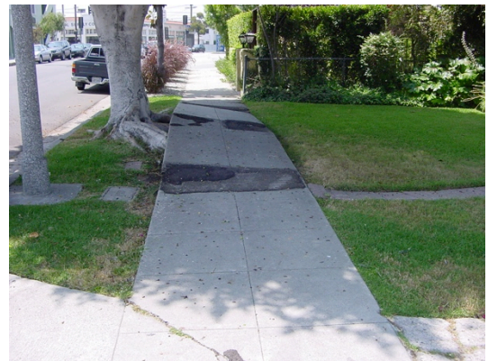
Uplifted sidewalk (Credit: Ryan Snyder)
